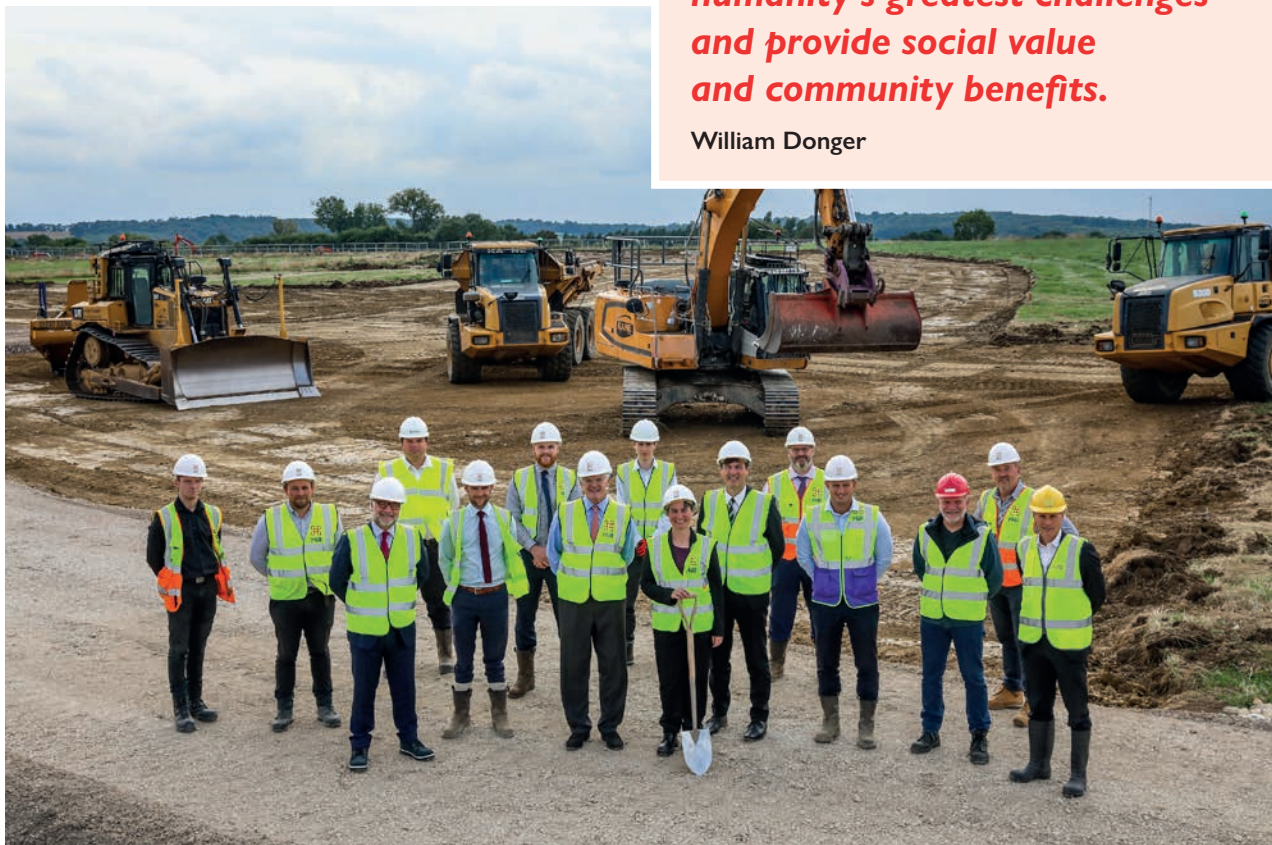
Ground-breaking ceremony: Zoe Hancock and William Donger are joined by Councillor Duncan Enright and Hill infrastructure and project team members – September 2021
